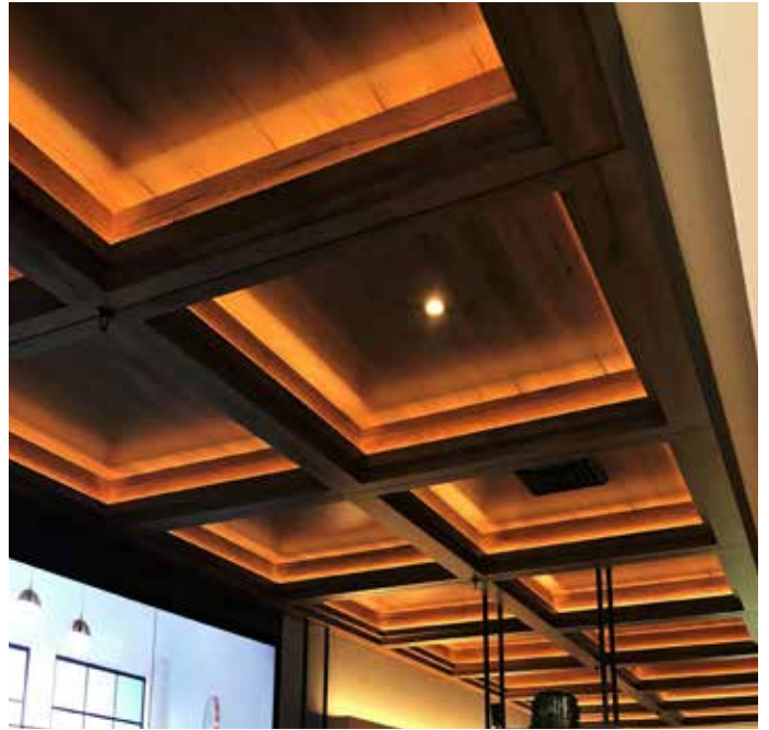
Installation method. Coffered ceiling using a combination of Ecolite Beams with MDF panels, featuring concealed lighting.
